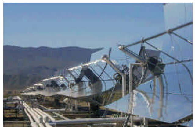
Direct steam generating parabolic trough test facility at the Plataforma Solar, Almeria, Spain
