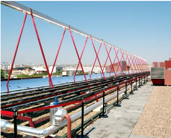
Figure 5.11 Fresnel process heat collector on the roof of Escuela Técnica Superior de Ingenieros, Sevilla
