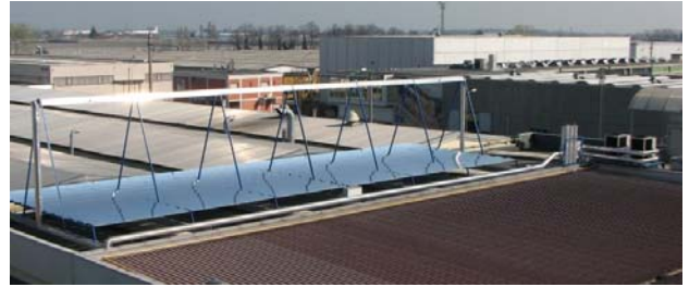
Figure 5.9 PSE Fresnel process heat collector powering two NH 3 /H 2 O absorption chillers (2006, Bergamo, Italy)
