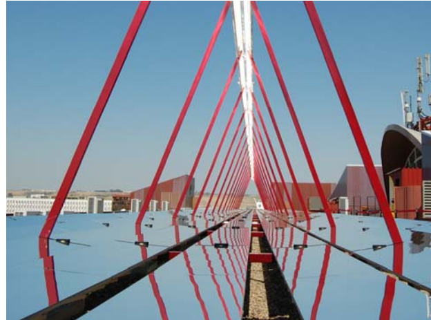
Figure 5.12 Fresnel process heat collector in operation
