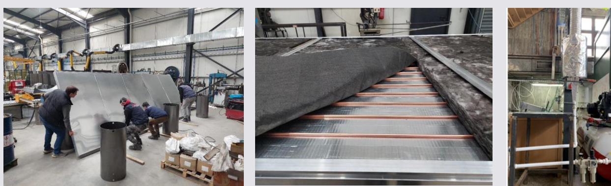
Figure 3: Solar thermal collector pilot construction phase & Laboratory test bed for the storage tank
