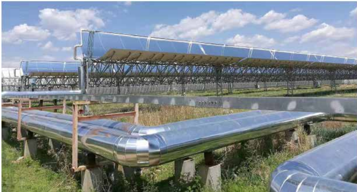
Fig. 4.2-6 China's First MW-scale Parabolic Trough CSP System (Yanqing, Beijing, IEECAS)
