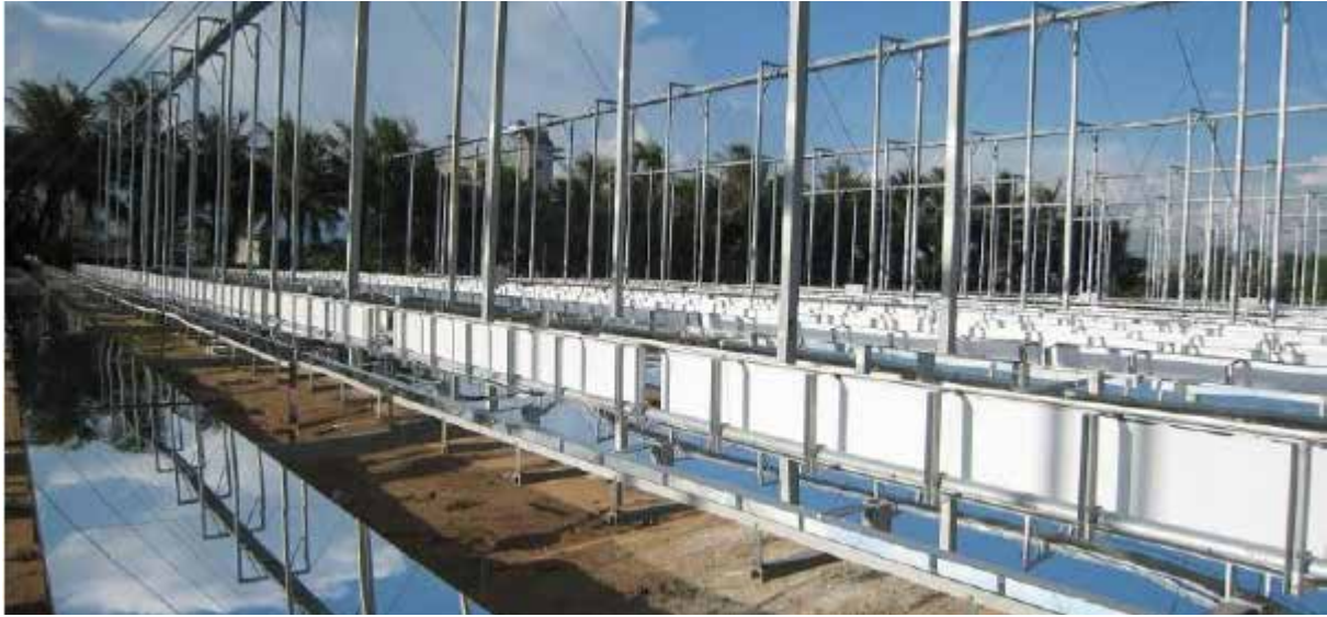
Fig. 4.2-3 Partial View of CSP Collector Field in Huaneng Nanshan Plant (Photo by Huaneng Clean Energy Research Institute)
