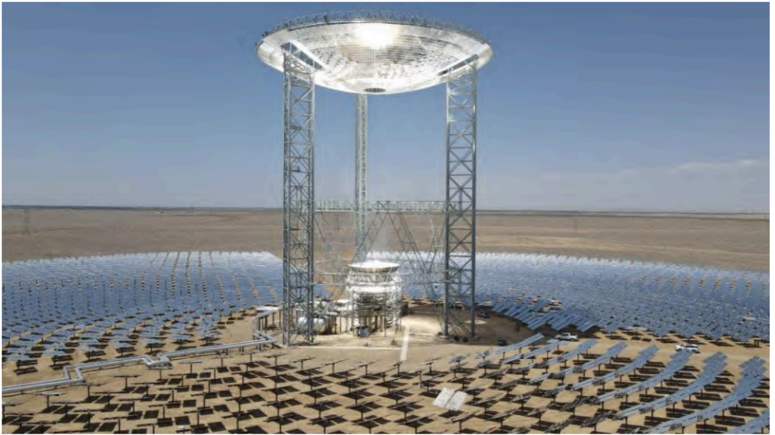
Figure 7: Secondary Reflection Tower System On-site Operating Photo
