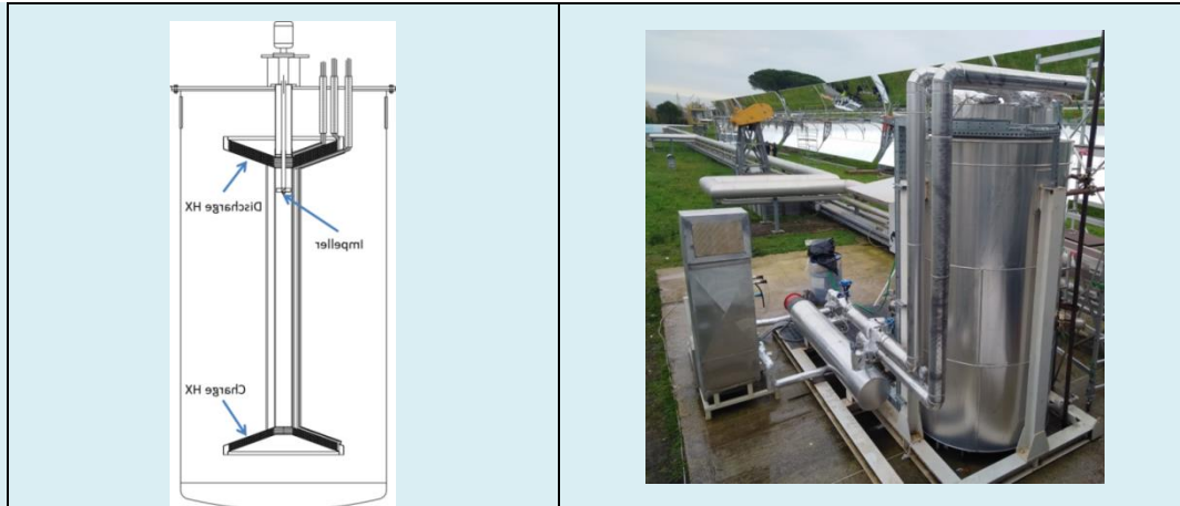
Scheme of the coupling CSP-TES-ORC and image of the prototype system installed at ENEA Casaccia Research Centre (Rome)
