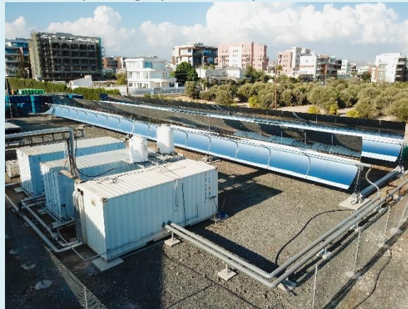
Figure 1: View onto the parabolic trough collector system with C-TES (Photograph ©Protarget AG)
