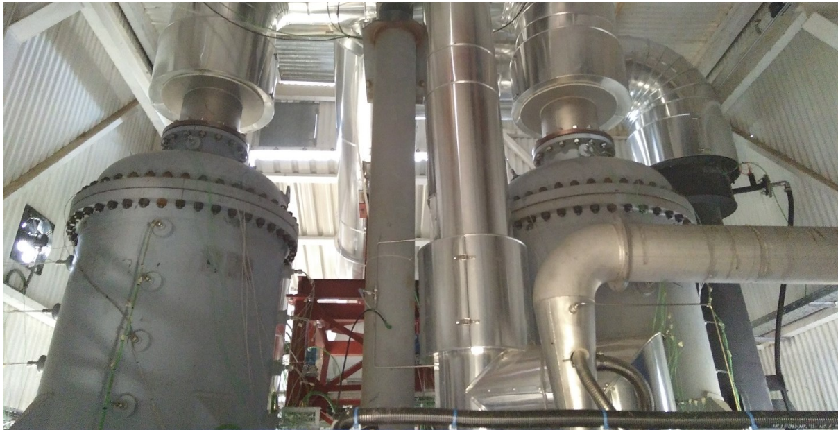
FIGURE 5. Picture of the two CAPTure regenerative heat exchange vessels and parts of air piping in the tower test room.
